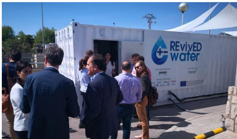
Figure 95. Outside of the container in which the integrated (R)ED-ED-RO system is installed. Photo taken during the inauguration and the visit at the plant on May 28, 2019 in Burriana, Spain.
