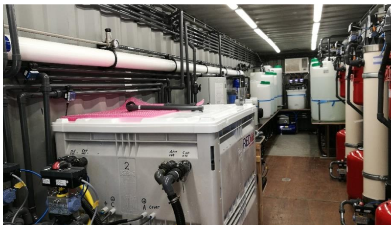
Figure 96. Inside the container. At the bottom left, the box containing the two stacks. Above the box, the RO pressure vessel. On the right, ultrafiltration systems.
