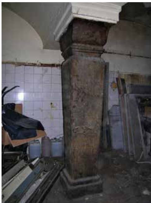
◇ Fig. 14 – Palermo. Palazzo Ferreri on Via Isnello, herm-shaped columns made of Monte Pellegrino stone on the ground floor prior to restoration (photograph by the author).
