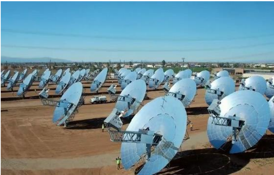
Figure 5. Maricopa Solar Project 1.5 MW in Arizona (source: http://www.feliciabellows.com )
