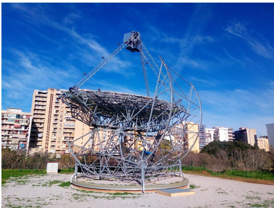
Figure 14. Supporting structure of the dish-Stirling reference system
