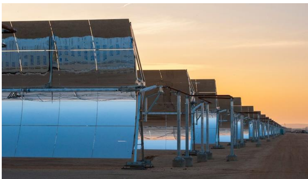
Figure 2. Mojave, a 250-MW parabolic trough CSP plant in California with a nominal annual generation of 617,000 MWh (Source: https://www.energy.gov/lpo/mojave )
