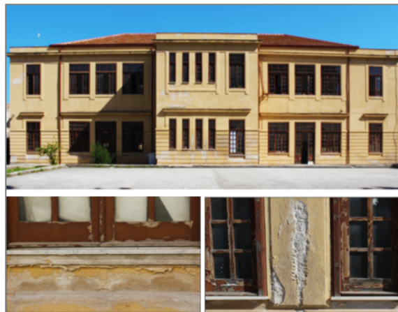
Fig. 2. Photographs of the back of the structure (top) and details of the windows (bottom), showing the poor state of maintenance.
