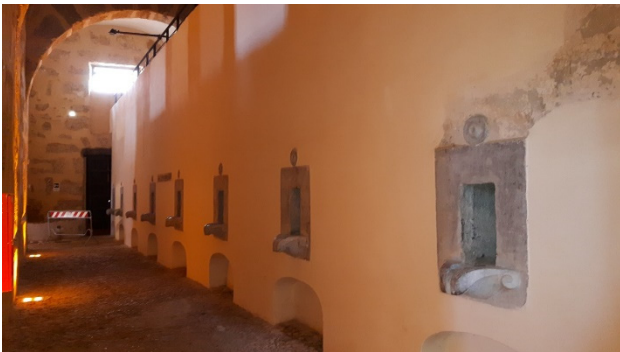
Figure 3. Interior of the “ Real Cantina Borbonica ”: the left aisle with the wine vats.
