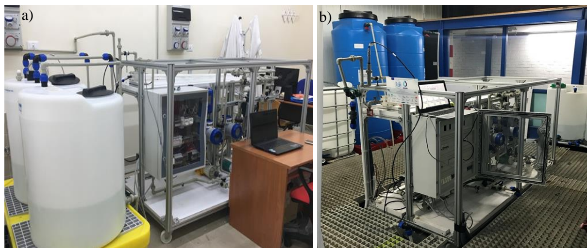
Figure 5. A picture of the novel proprietary crystallization reactor tested at the Brine Excellence Center laboratory of University of Palermo (a), then installed and operated at the premises of Plant One (Botlek, Rotterdam, NL) (b).
