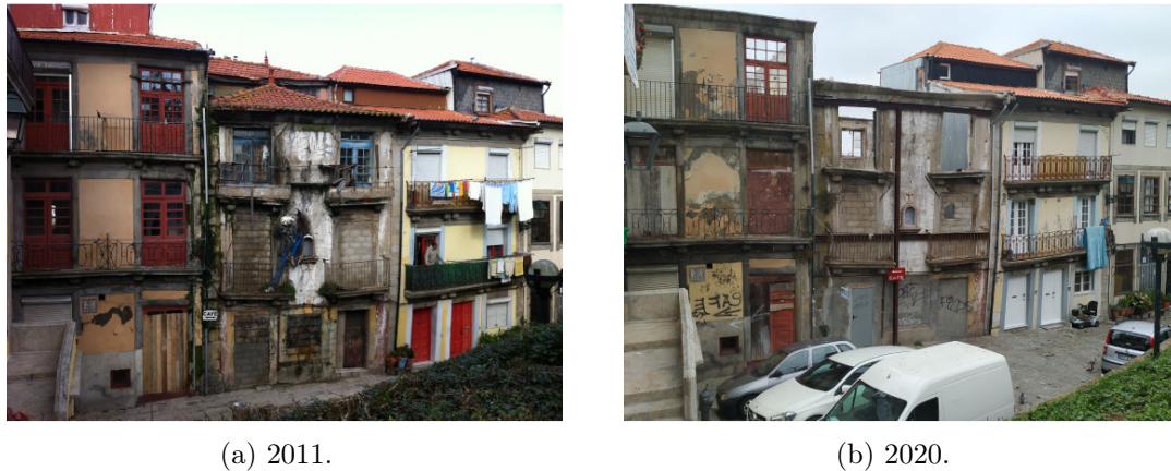
Figure 5.12: Sé Urban Rehabilitation Programme, public-owned buildings waiting for intervention, Pena Ventosa street. The alarming state of building disrepair has got worse with time. Source: photo 5.12a by ecudiélle licensed under CC BY-ND 2.0 and photo 5.12b by author.
