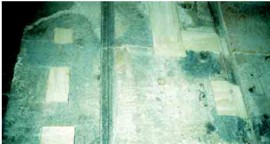
Fig. 14 Palermo, 'Palazzo Belmonte-Riso'. Detail of the outside façade face wall during some of the phases of the yard
