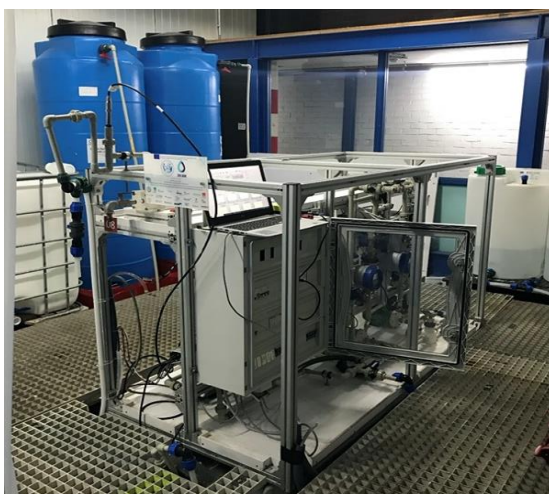
Figure 8.3. A picture of the MF-PFR prototype installed and operated at the premises of Plant One (Botlek, Rotterdam, NL).
