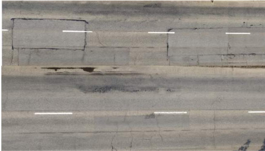
Figure 9. Cropped sections of the pavement model's surface (( top ) image shows a cracked and rutted sub-section and the ( bottom ) image shows a sub-section with depression, cracking and rutting distresses).
