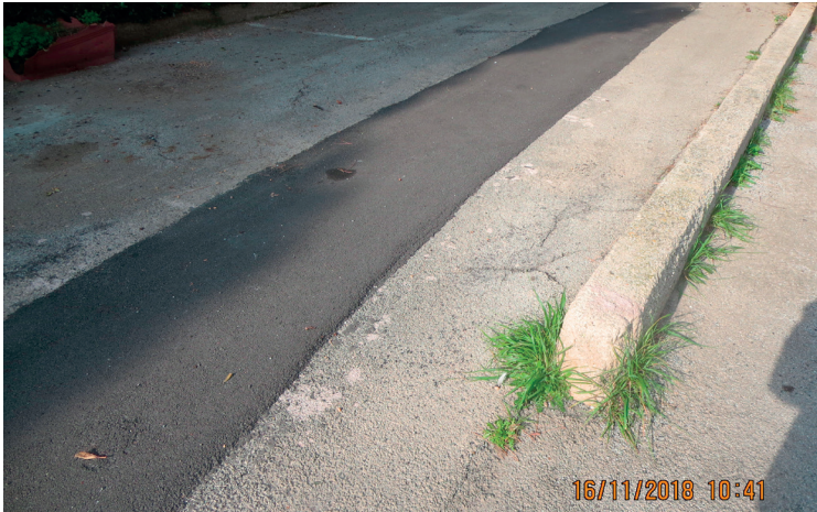
Photo 8. Destruction of the asphalt of the road for the lifting operated by the roots.
