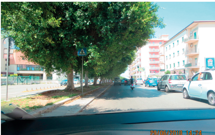
Photo 2. Traffic divider too narrow with damage to the wall and the sidewalk (torn) and risk of lifting the road surface, already evident in some points. The plant species present is Ficus benjamina .
