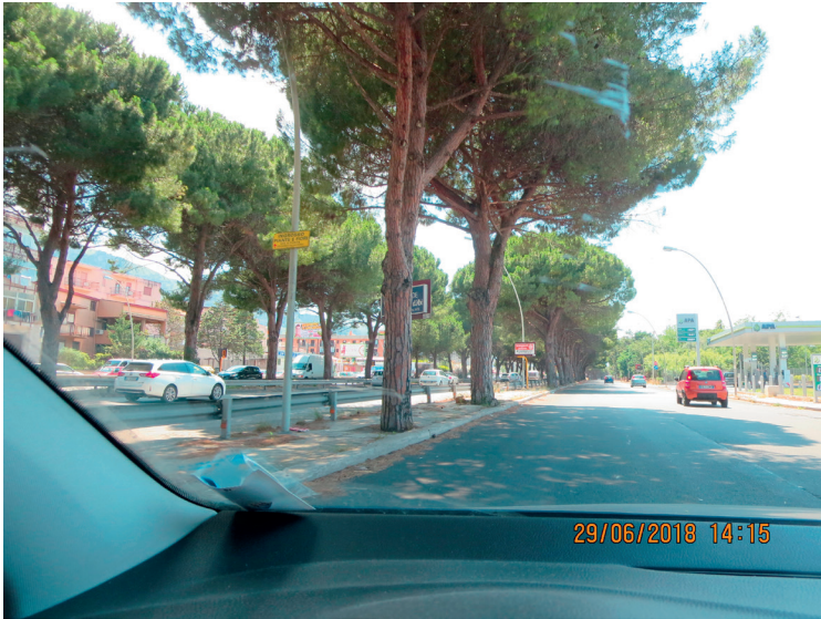
Photo 3. Traffic divider with Pinus pinea whose roots lift the asphalt and the managing body is forced to redo the bituminous mat frequently, with considerable running costs.
