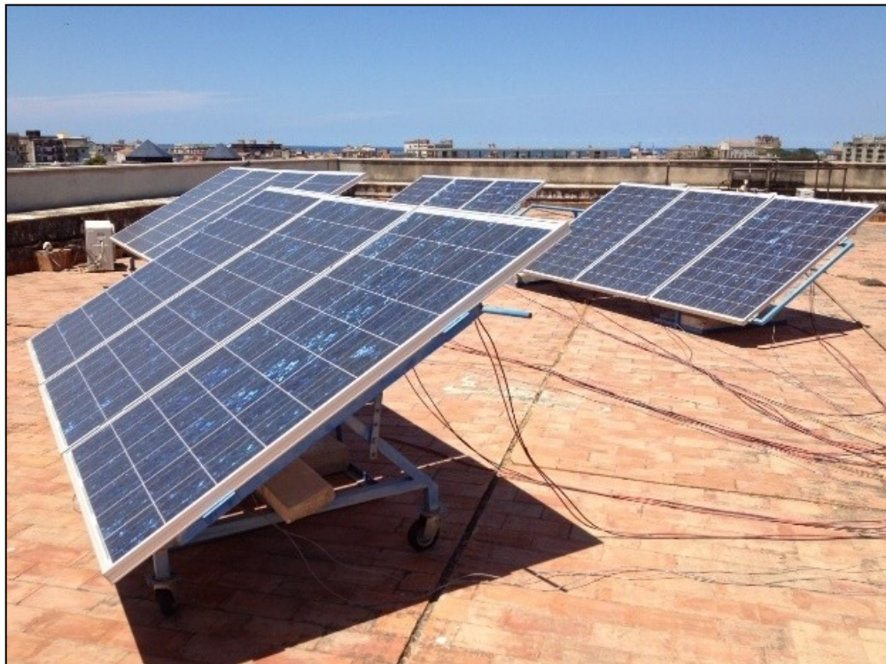
Figure 7. Experimental system with panels individually connected to DRS.
