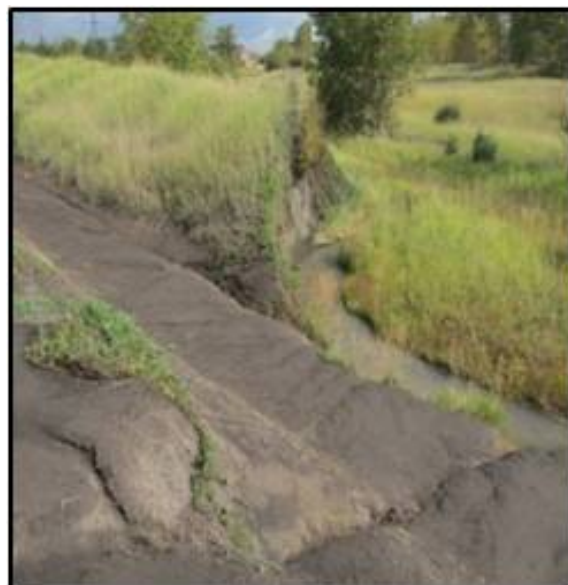
Fig. 4. Washout the soil in the Tikhaya River
