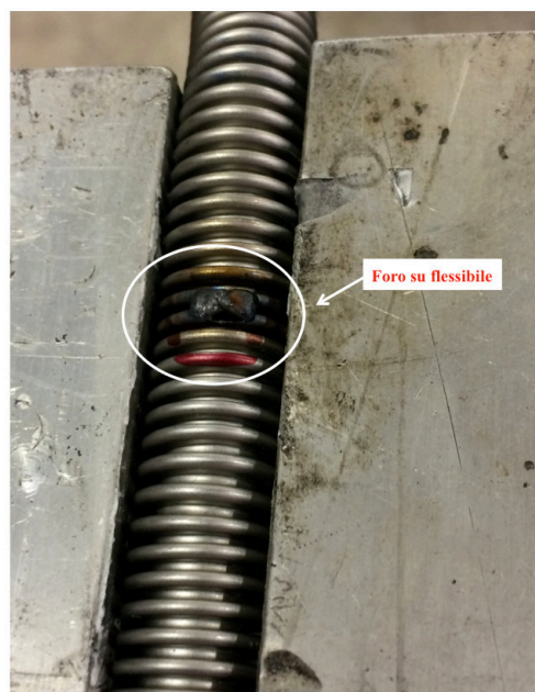
Fig. 2 – Example of damaged flexible
