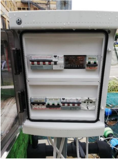
Figure 5.13: Electrical panel in the plant area. It is possible to see a master switch, the switch for the monophasic plug, the two switches for the pumps and a general switch followed by single ones for the flowmeters.
