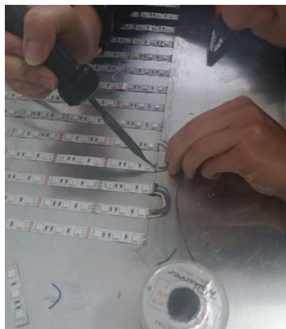
Figure 3.8: Installation process of RGB LED strips (KWB 5m 5050 RGB IP44) on aluminium panel in order to make LED panel.
