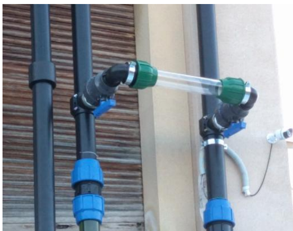
Figure 5.6: Modified degasser, at 5.7 m from the ground.
