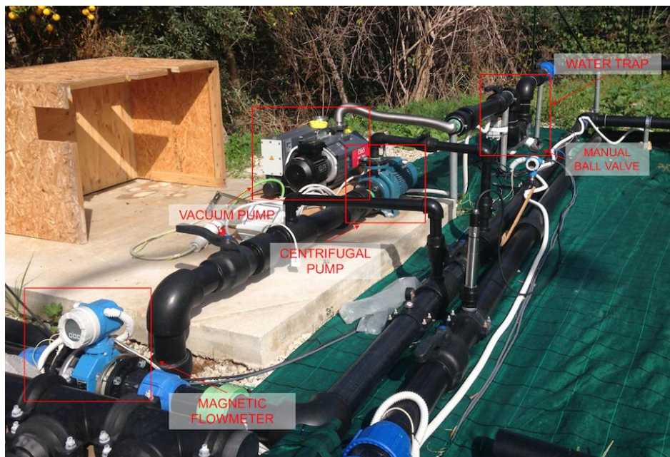
Figure 5.10: Detail of the circulation/input system in which a centrifugal pump and a vacuum pump are shown.
