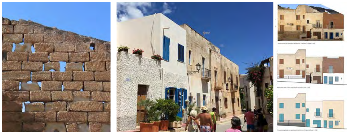
Fig. 8-10: Main risks in Egadi Islands: wind erosion and marine aerosol; introduction of colors extraneous to tradition (white, blue); partial maintenance and transformation of the facades according to the property regimen.
