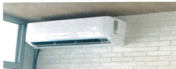
b) PV - Air conditioner: internal unit
