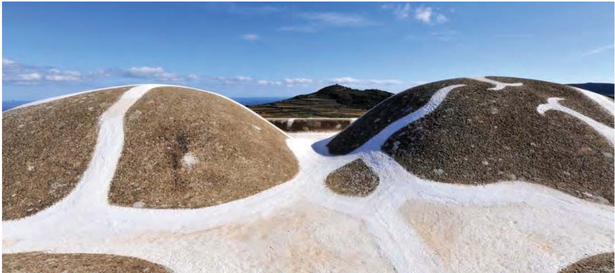
Fig. 14: Finishing of a stone vault by means of a natural hydraulic lime layer. Cracks were closed by means of fresh mortar.
