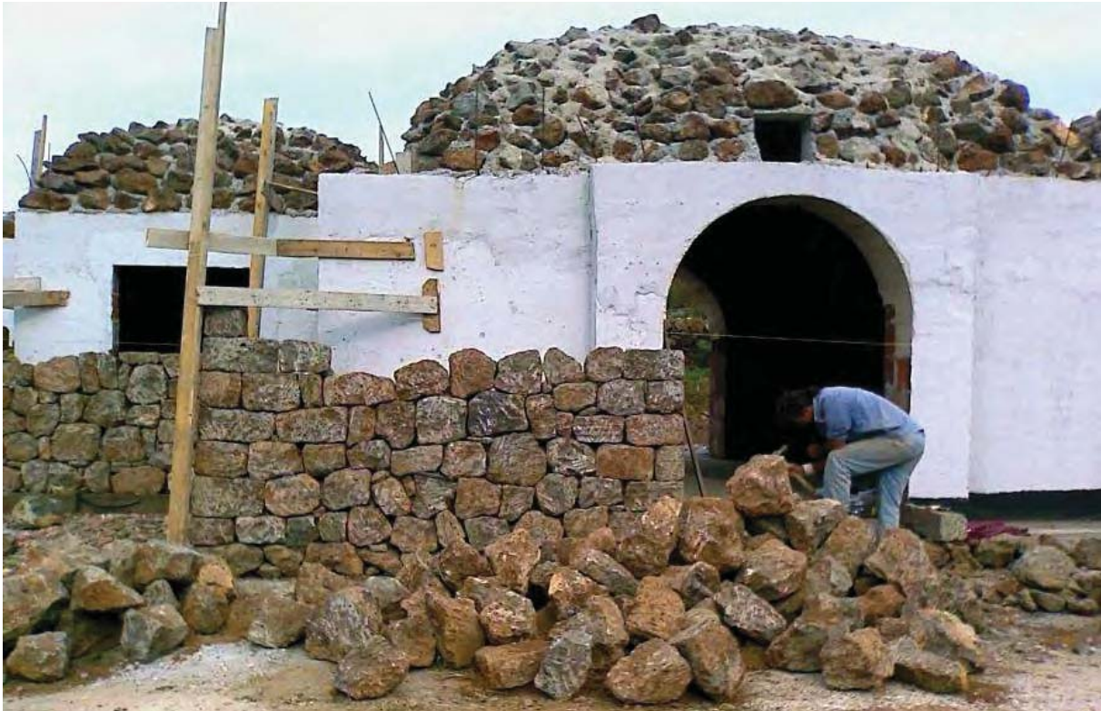
Fig. 16: The exterior of a modern dammuso , built using contemporary constructive technologies, is then covered by natural islander stones to simulate the traditional aspect of the building typology.
