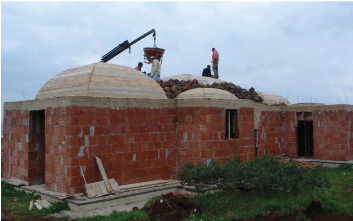
Fig. 15: Construction of a modern dammuso using contemporary constructive technologies. According to the Pantelleria Building Regulations, aspect, shape, and dimension of a traditional dammuso are respected. Moreover, the vault is realized by means of real stones.
