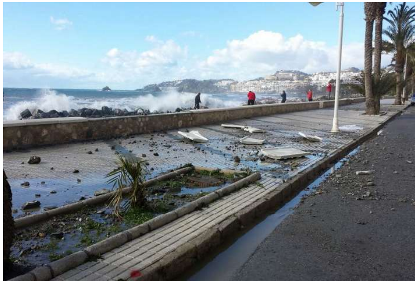
Figure 2. Severe damage after a western storm in winter 2015 at the Reina Sofia Promenade (Almuñecar), photo by europapress.
