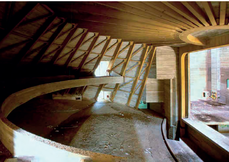
Figura 9. El interior de la sala mayor en estado de abandono. Foto de Giovanni Palazzo, (2004) / Figure 9. The interior of the main auditorium in a state of neglect. Ph. Giovanni Palazzo (2004).
