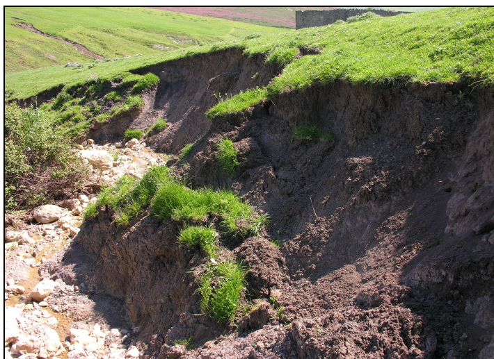
Figure 5.17. Bank erosion causing river walls collapse (12.05.2011).
