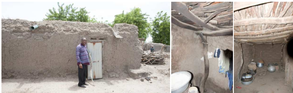
Figure 18. Exterior and interior of a hut with a cover in raw earth where the supporting wooden structure is highlighted.
