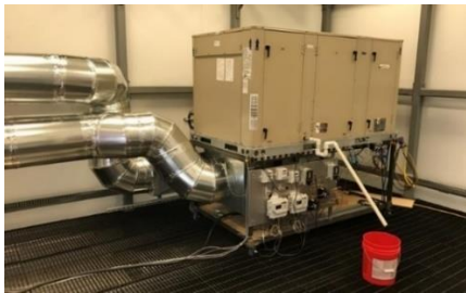
Figure 1. Packaged rooftop air conditioning unit installed at Herrick Laboratories
