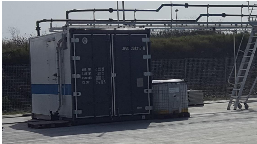
Figure 30 – The FC container set-up installed inside the INGRID demonstrator.
