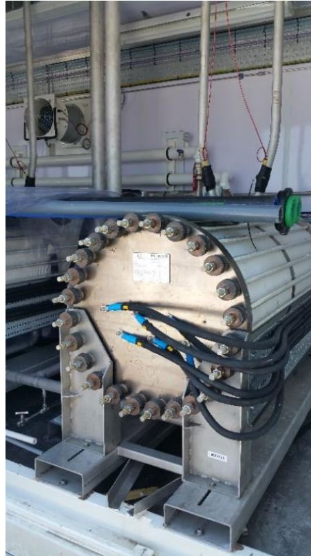
Figure 27 – One of the four cell stacks installed inside the WE.
