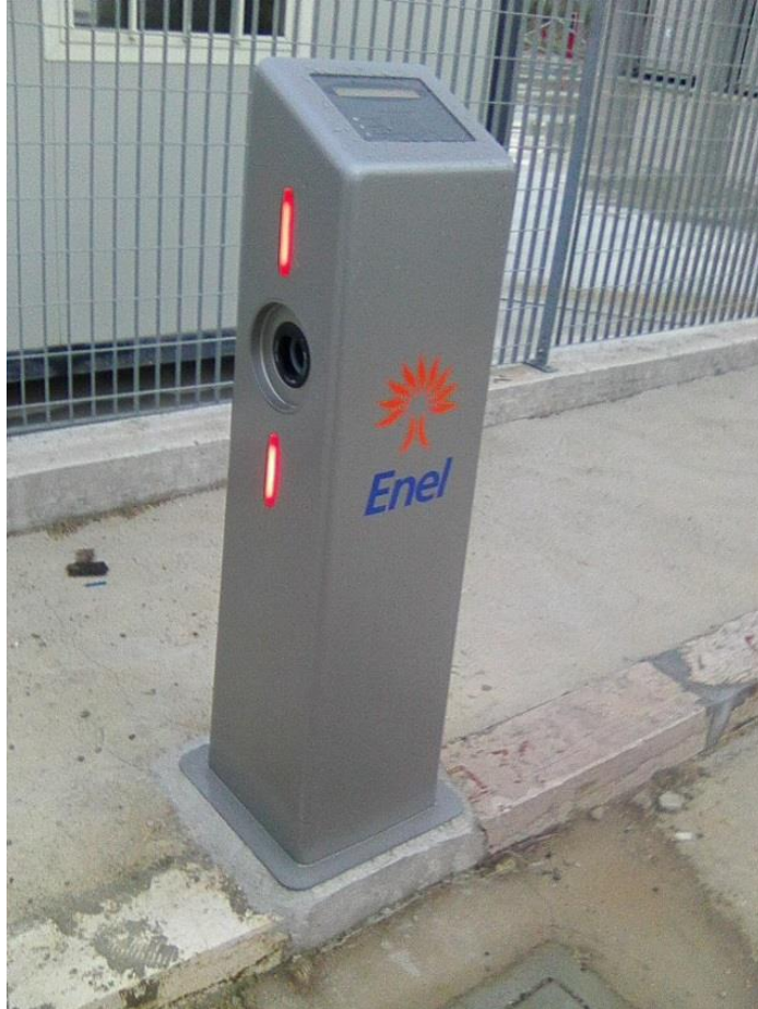
Figure 33 – The EVRS installed inside the INGRID demonstration site.
