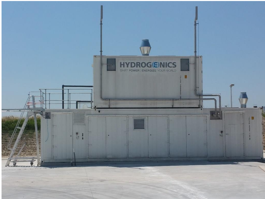
Figure 28 – The complete set-up of the WE deployed inside the INGRID plant.
