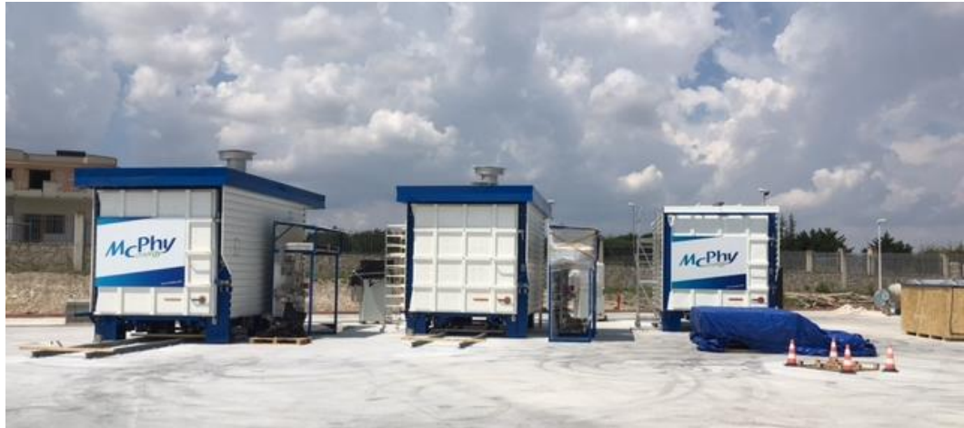
Figure 32 – The complete HSS systems installation inside the INGRID demonstration site.
