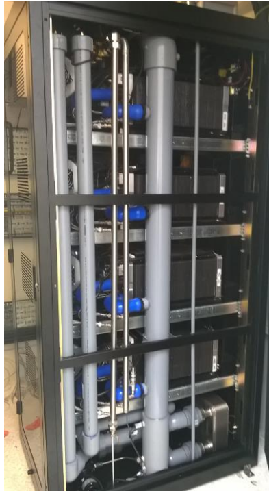
Figure 29 – The cells rack installed inside the FC.
