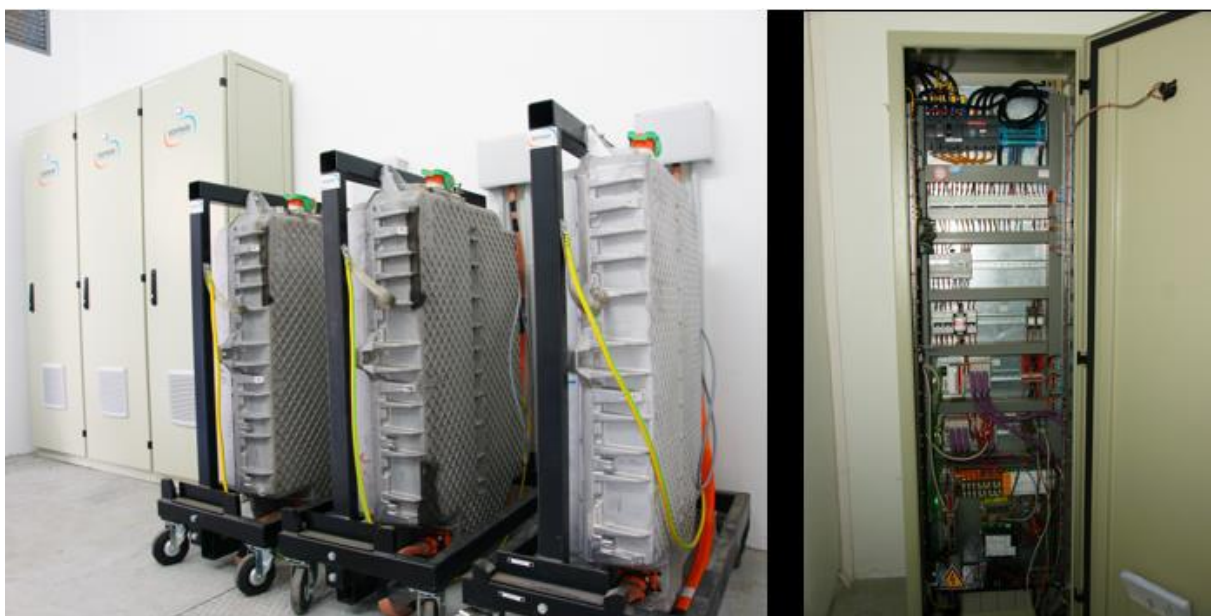
Figure 53 – Picture of the installed storage system proposed in the ELSA project.
