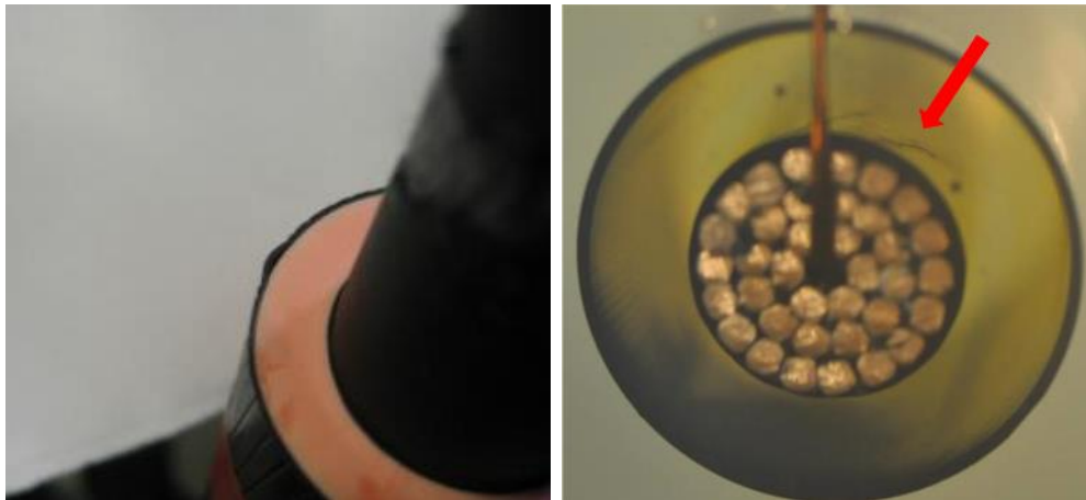
Figure 1-7. Defects on cables
