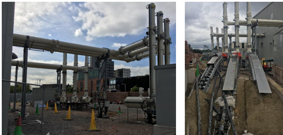
Figure 6-16. Underground cables at 400 kV and GIS Termination
