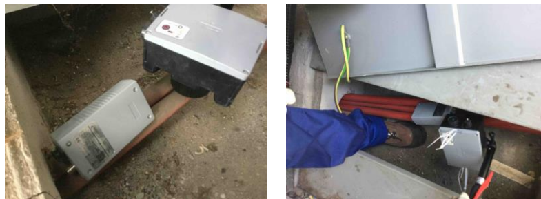
Figure 6-71. Pry-Cam Portable placed on cables
