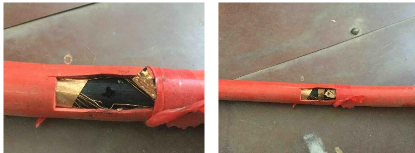
Figure 4-1. Defect in MV cable specimen
