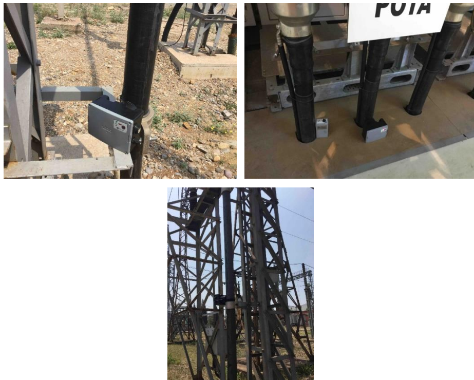
Figure 6-53. Pry-Cam Portable placed on cable close to the GIS and outdoor termination
