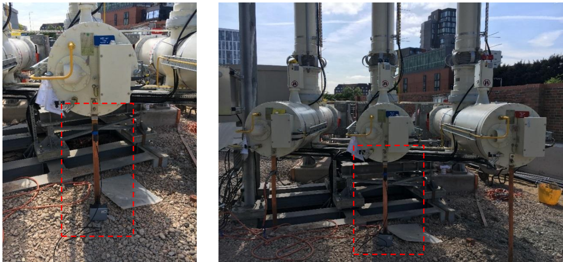
Figure 6-19. Pry-Cam Wings installed on the earth connection of the GIS cable sealing end.
