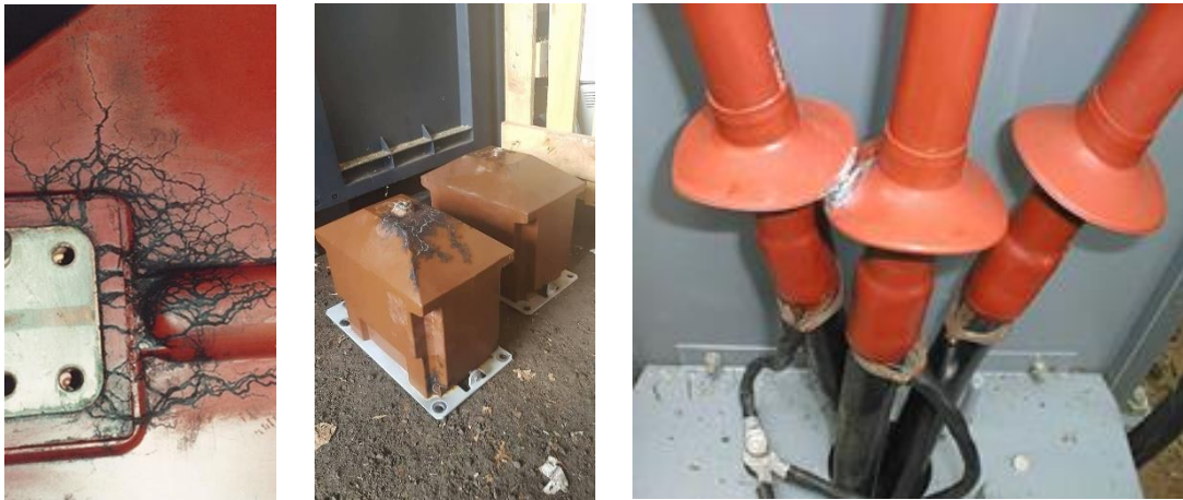
Figure 1-10. Surface discharges effects
