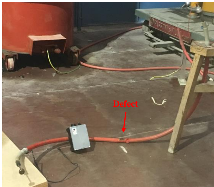
Figure 4-3. Pry-Cam Portable placed on cable close to the defect
