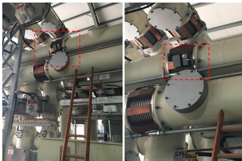
Figure 6-27. Pry-Cam Portable placed on the earth connection of the GIS switchgear.
