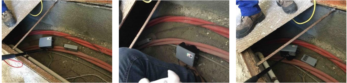
Figure 6-67. Measurement performed on cables close to the switchgear box
