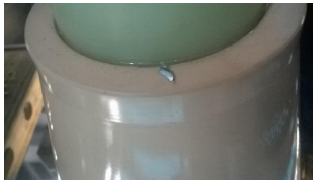
Figure 1-15. Metallic protrusion inside 380 kV cable termination
