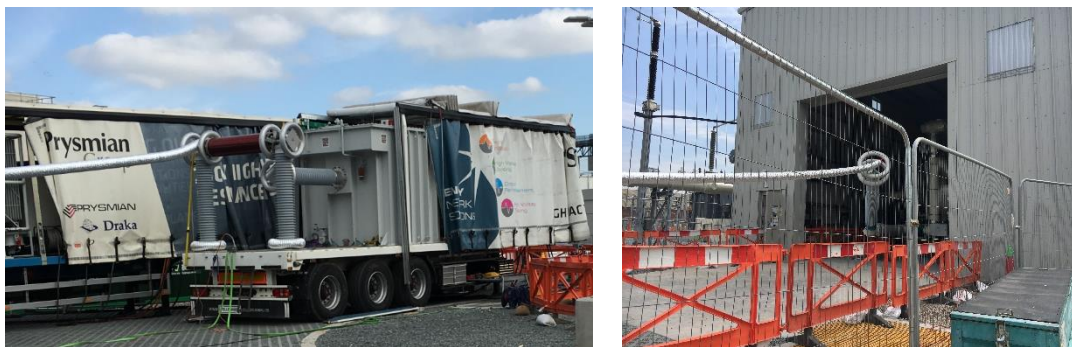
Figure 6-15. AC resonant system connected to the GIS switchgear system
