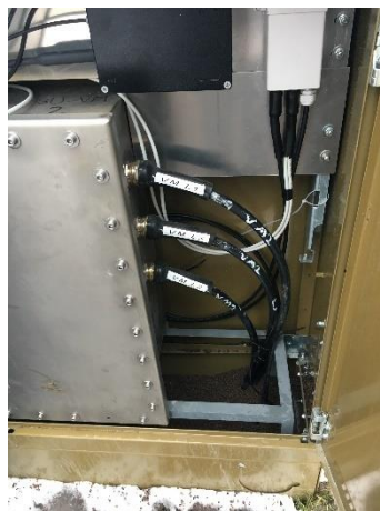
Figure 6-37. Pry-Cam portable placed on cross bonding leads inside pillar
