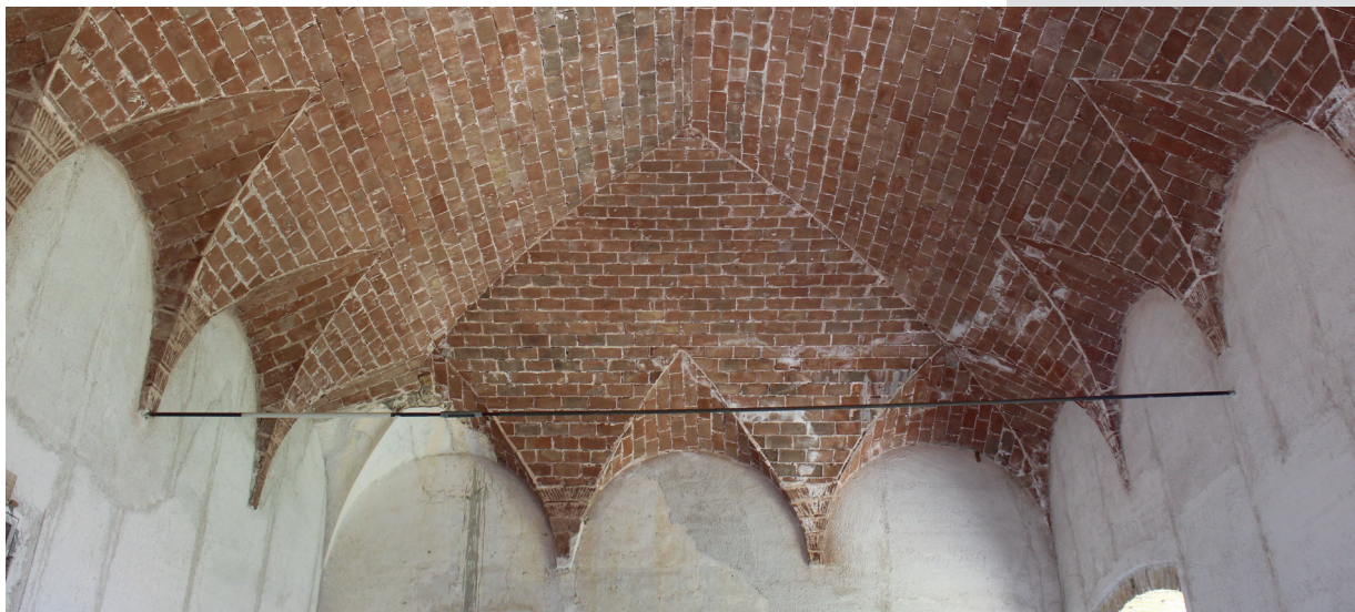
Figure 6. Realization of a tiled cloister vault with lunettes, taking place a collapsed stony one.
