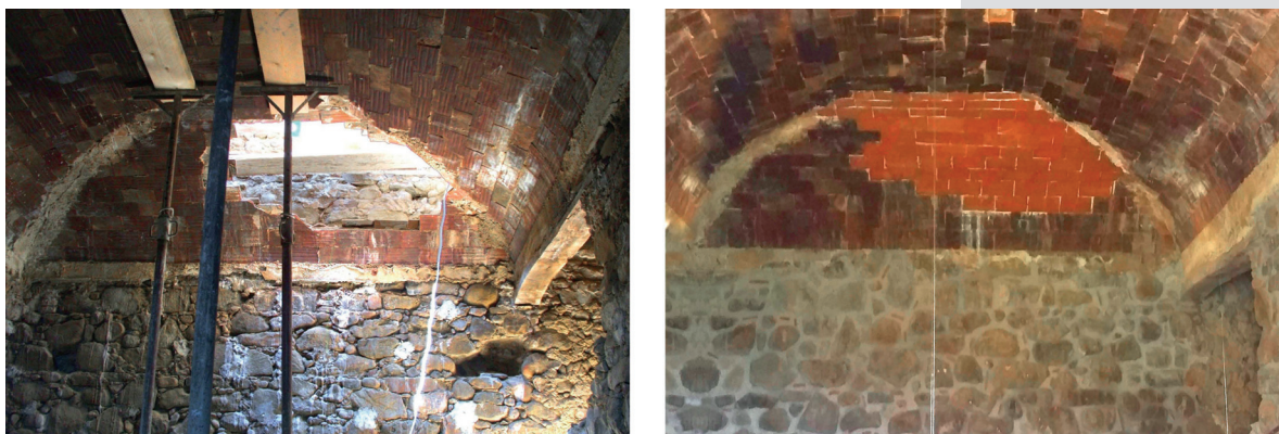
Figure 3. Reconstruction of a small portion of a broken down tiled vault.
