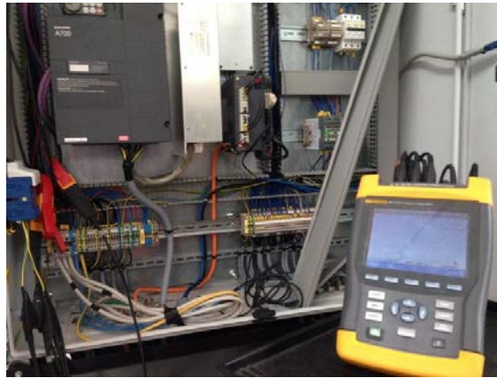
Fig. 2. Cabinet of the utilized machine during the measurements showing current clamps and tension alligator clips.
