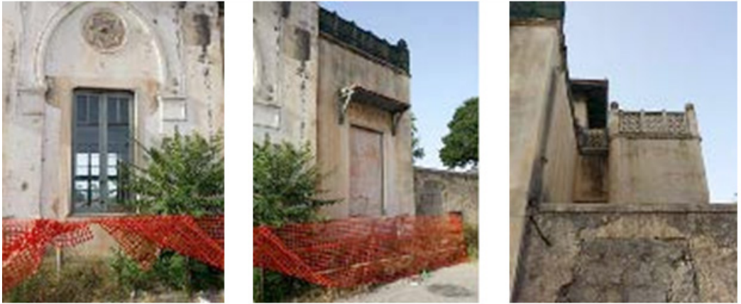
Figure 4a, 4b, 4c, Stand Florio, analysis of the building degradation.
