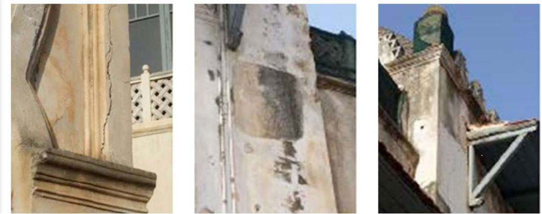
Figure 6a, 6b, 6c, Stand Florio, analysis of the building degradation.
