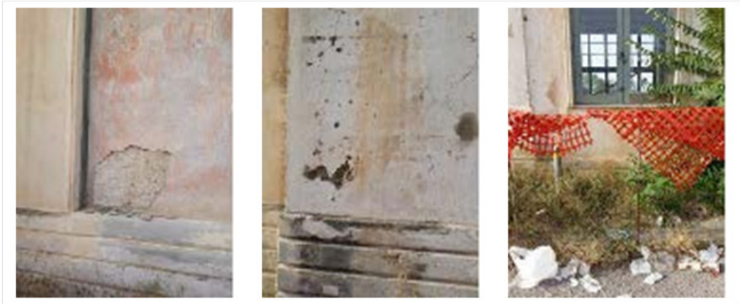
Figure 5a, 5b, 5c, Stand Florio, analysis of the building degradation.
