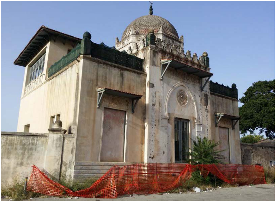
Figure 3, Stand Florio, Palermo, Sicily. The construction degrade the south facade
