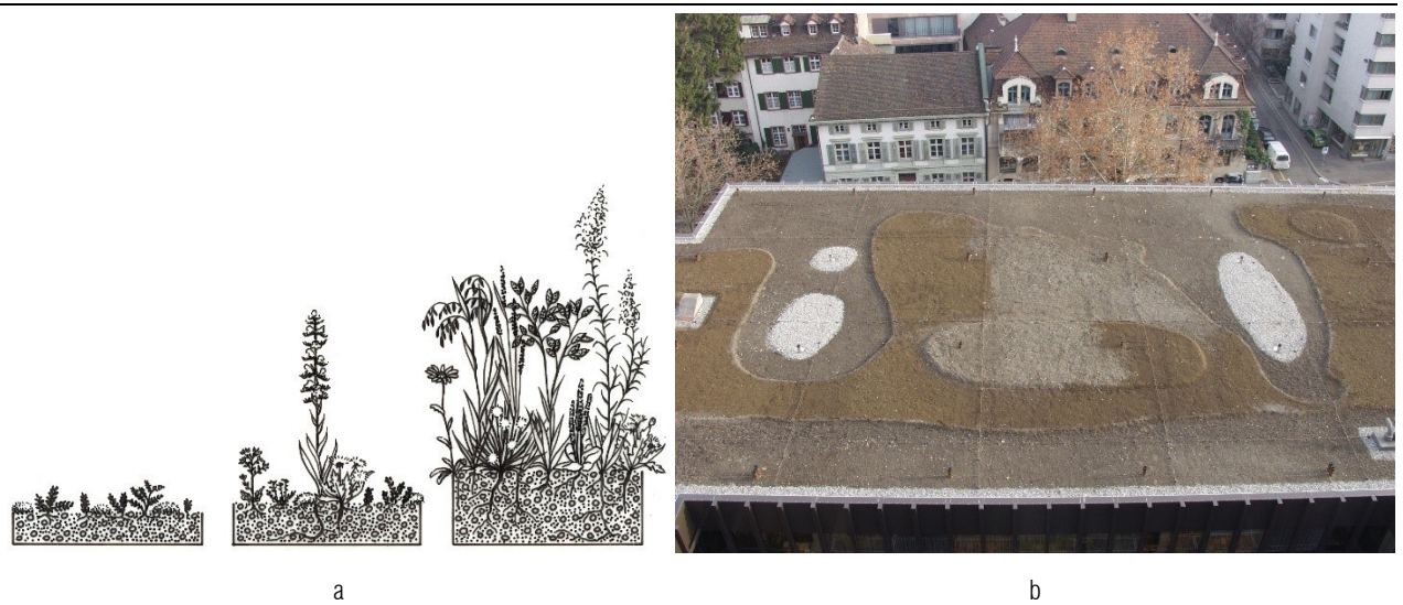
Figure 4. a) Substrates of different thickness (6, 12, 20 cm) used to accommodate different biotic communities on the roof of the Cantonal Hospital in Basel (Klinikum II). Design Stephan Brenneisen, University of Applied Sciences Zurich (ZHAW). b) Klinikum II roof from a bird's-eye view perspective (photo Stephan Brenneisen).
