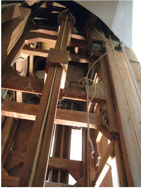
Figure 18. The masts carrying the four rising discs of the table can slide with respect to rectangular frames sliding along vertical rails gouged in the fixed scaffolding (see also Fig. 12 and upper left corner of Fig. 15).
