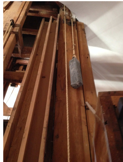
Figure 15. One of the four traction ropes on the corner for the lifting of the central frame. On its side, another rope carries one of the four leaden counterweights that were hung to facilitate the frame hoisting.
