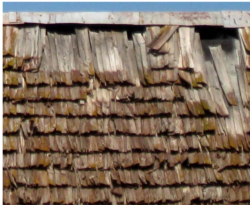
Figg.2,3: On the left: the walls cladding of the wooden boards is one of the most frequently replaced elements. Lack of maintenance of the external cladding can lead to irreversible degradations. On the right: damage to the outer covering of the roof accumulates water into the attic area, increasing the moisture level (over 20%). This disruption can cause fungal attacks to the roof structures.
