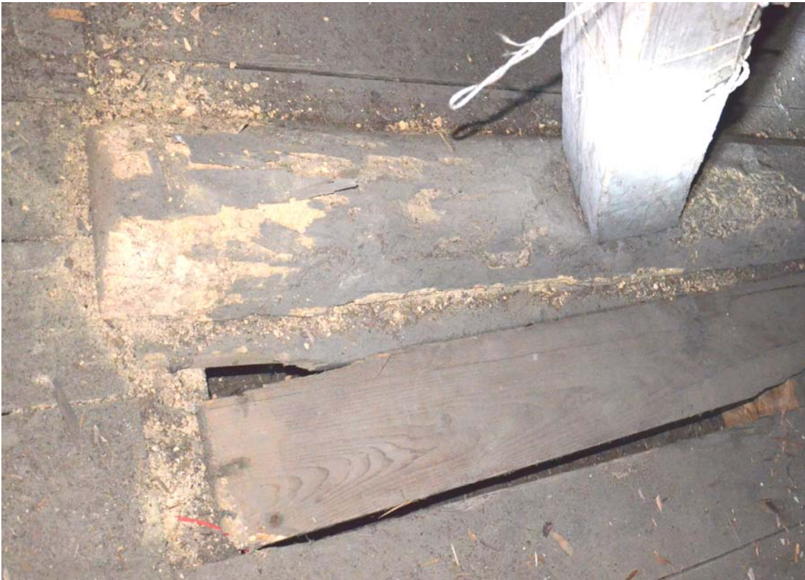
Fig.6,7: Example of wooden beams irreparably damaged; even a small number of holes can hide a very serious state of deterioration.
