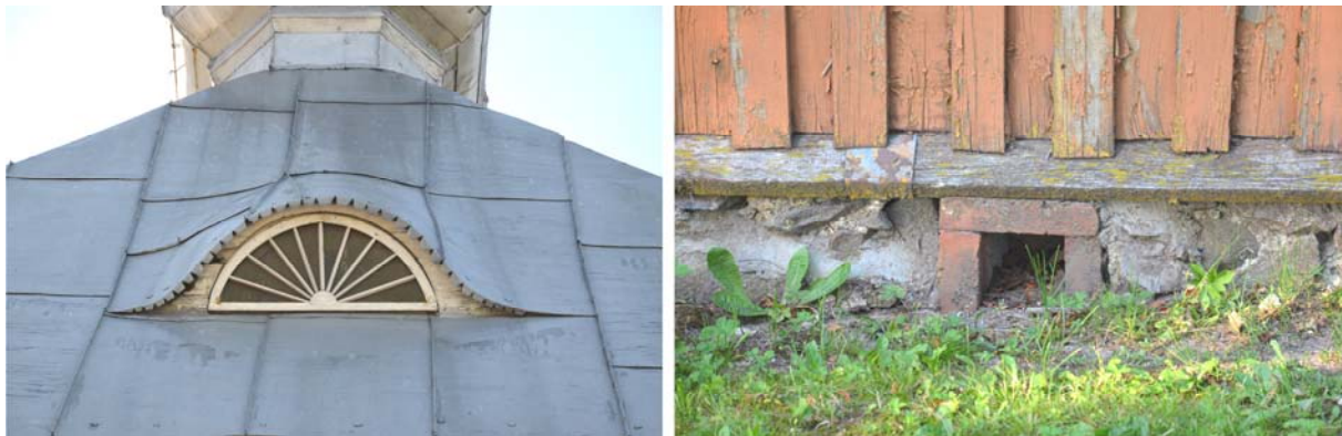
Figg. 12,13: On the left: in the attic area the local workers during the construction work preferred to install windows that guaranteed a good ventilation of the roof structures, during the year; on the right: in the past, it was preferred to open holes directly in the foundations, to ensure a good ventilation of all foundation zone.
