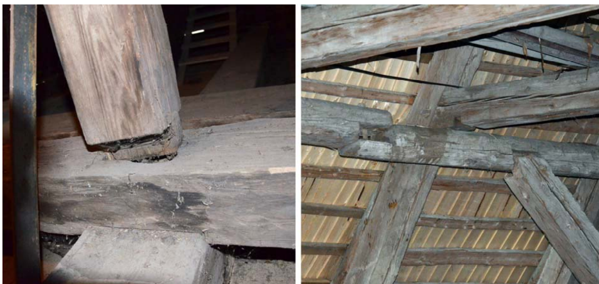
Figg. 8,9: On the left: a disconnection between the king-post and the tie beam. On the right: all nodes of the roof structure are disconnected, due to the shrinkage cracks.
