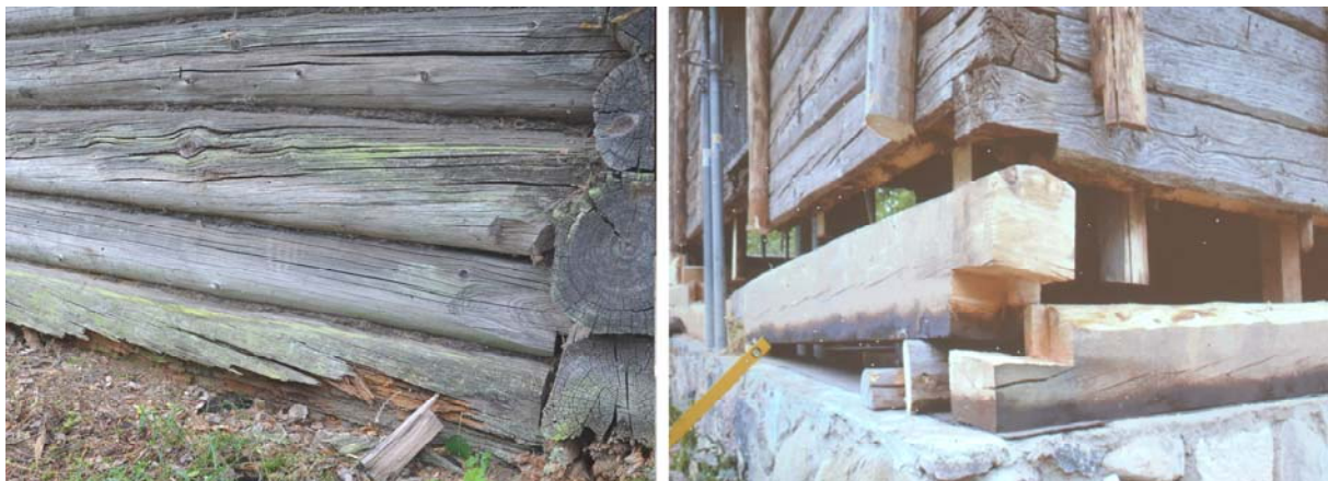
Fig. 10,11: On the left: the lower wooden wall trunk is in a direct contact to the ground, deteriorating by soil moisture. On the right: in case of total damaged logs, trunks can be replaced raising the wall structure and removing the damaged parts.
