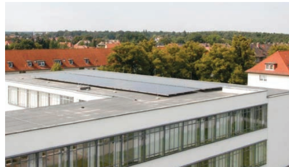
Photo 13 - Black micromorph silicon PV panels installed flat on the roof of Bauhaus Foundation Building, Dessau
