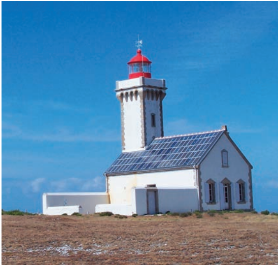
Photo 5 - Phare de Poulains, Belle-Île-en-Mer (Sauzon), built in 1867, renovated in 2006: view of the building-integrated solar plant of 3 kW
