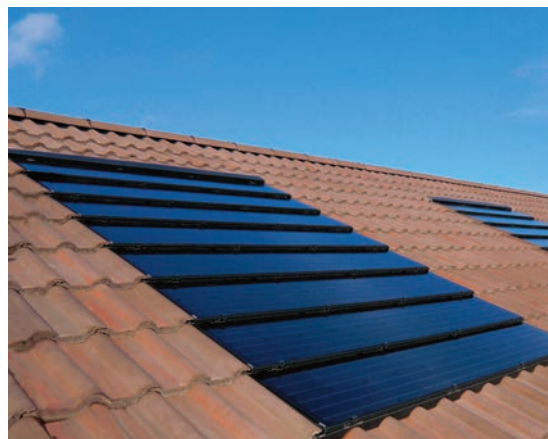
Photo 5 - Building-integrated PV system, installed as part of a pitched roof weatherproofing layer
