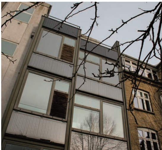
Photo 6 - Det Gule Hus, Esbensen Engineering, Aalborg, 2000: retrofitted façade with PV-integrated sun spaces
