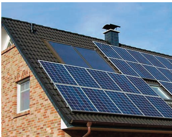
Photo 4 - Building-added PV system, installed on a pitched roof with independent supporting structure
