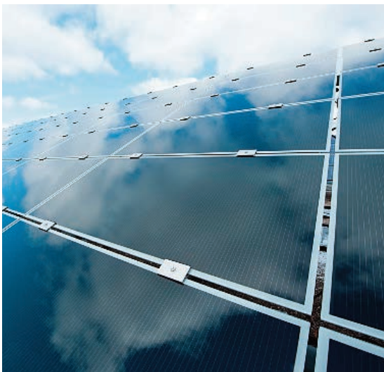
Photo 17 - Example of a Cadmium Telluride photovoltaic array
