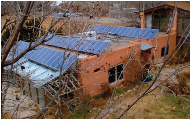
Photo 6 - Example of subjugation : PV system retrofitted on a flat roof
