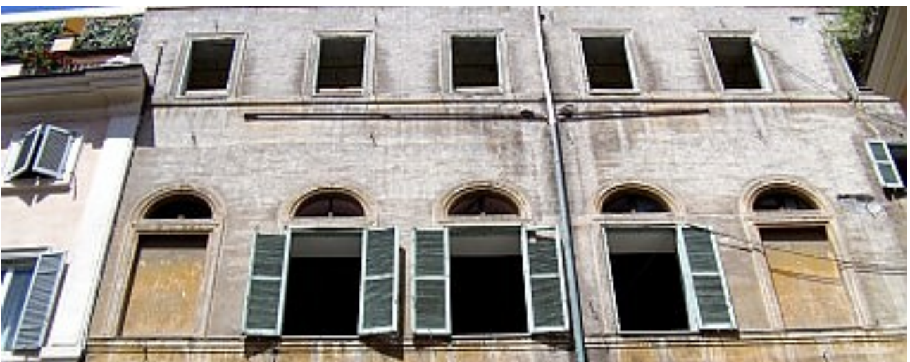
The view of the Angelo Mai complex façade from the street via degli Zingari
