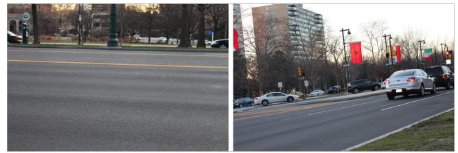
Fig. 1. Full scale rut depth: depression in the wheel path.
