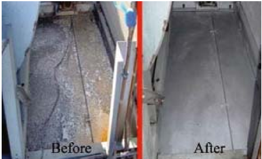
Figure 8. Duct before and after the treatment.
