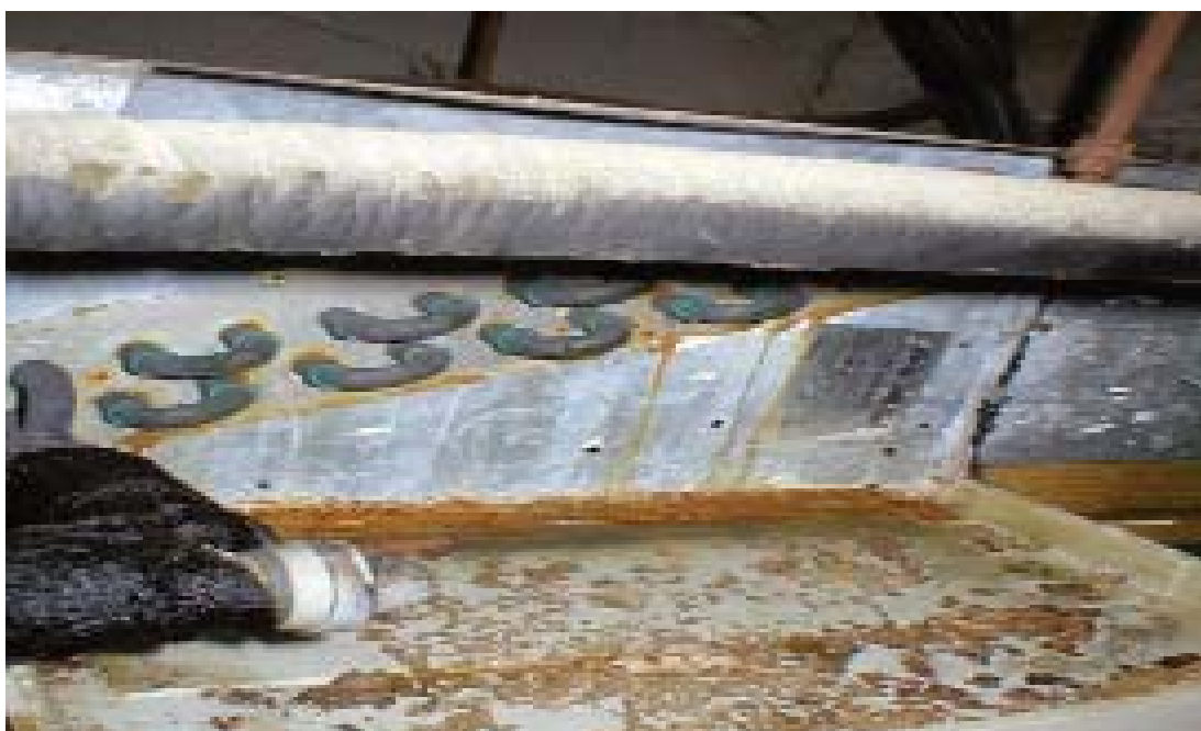
Figure 4. Encrustations in heat exchanger.
