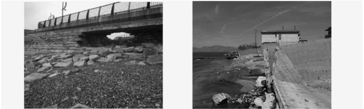
Figure 1 – Collapse of coastal defences in Portsmouth (left) and coastal erosion and flooding consequences on a shoreline house in Litorale Domitio (right)
