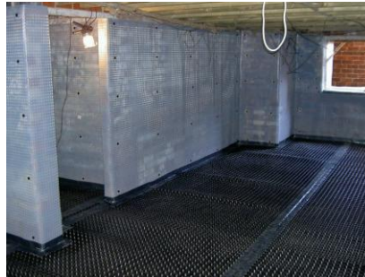
Figure 2.1: Basement floor and walls covered with plastic render.
