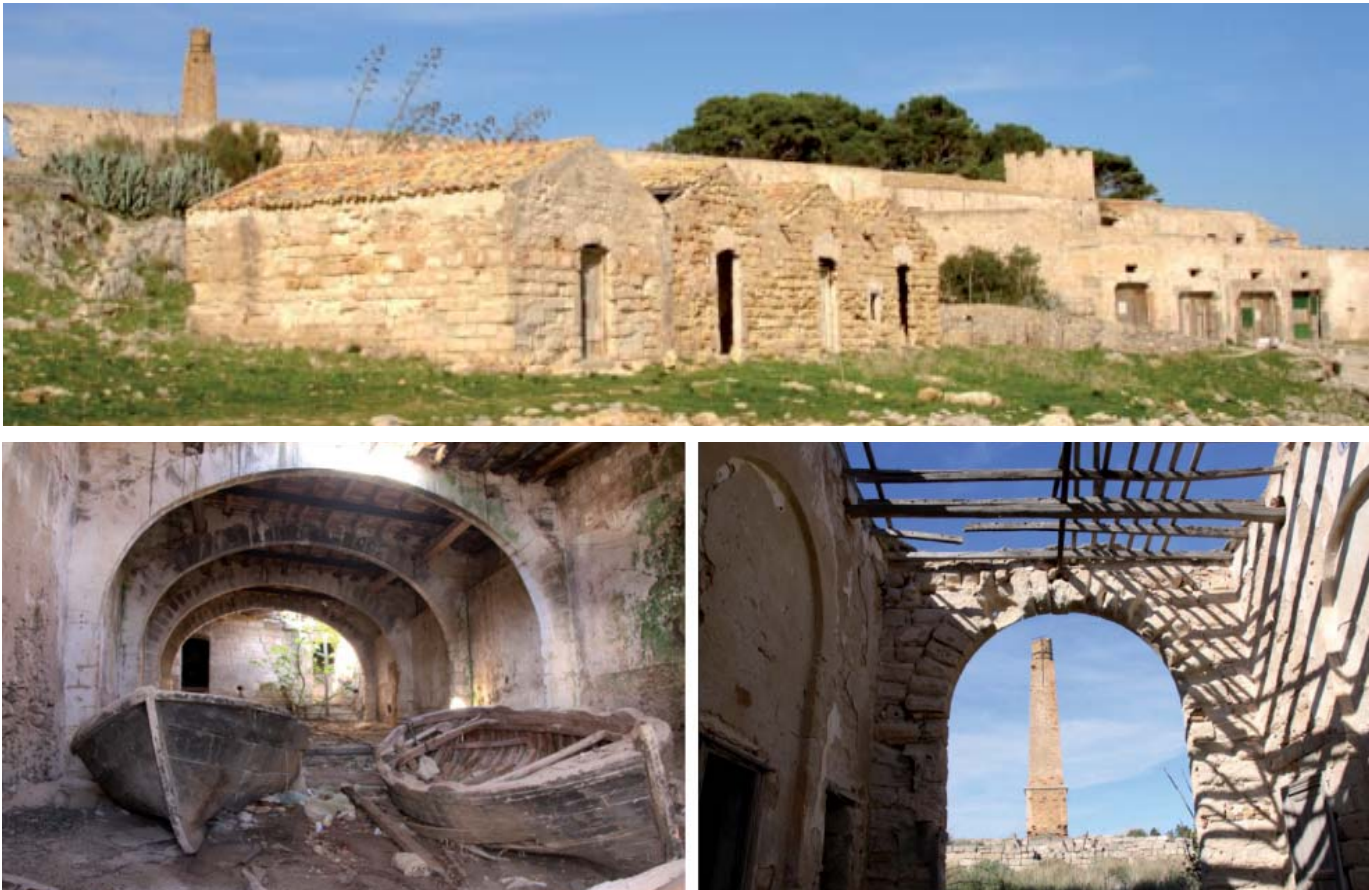
Fig.10 – Tonnara of Secco, San Vito Lo Capo; Fig. 11 – Tonnara of Secco: a collapse on the trizzane, with the ancient boat, and a view on the internal court
