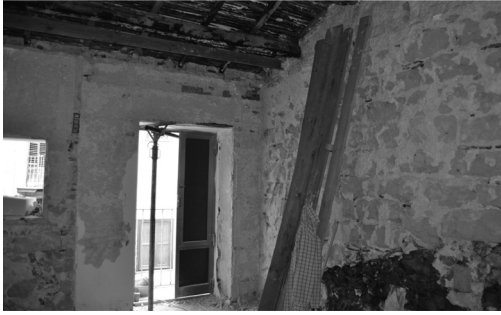
Figure 4. Third storey of a historical building in via Spinuzza a Cefalù; on the lower right, the wall in adobe (photo by M. Caliò & M. Guercio, 2010).
