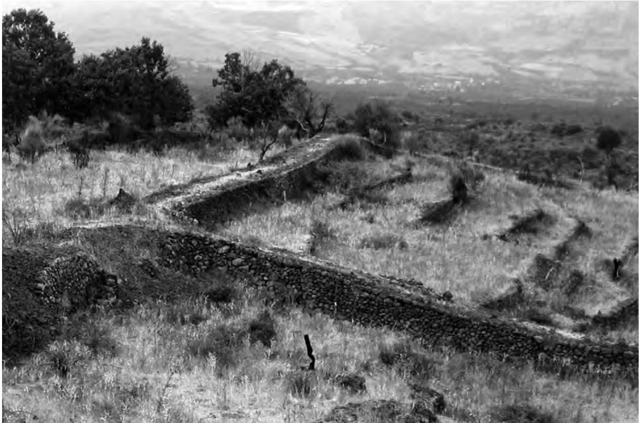
Figure 4. Abandoned terraces recovered by plant renaturation processes and increasing of stability problems of dry-stone walls (N-Sicily).
