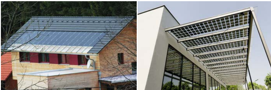
Fig. 10.23 a-b In these the buildings photovoltaic modules in laminated safety glass were installed on the roof by Ertex Solar. Left: family House in Thyrnau (Austria). Right: WKÖ head-quarter (Geneva).
