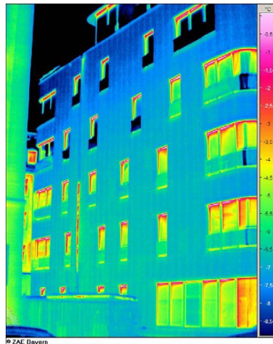
Fig. 10.11 Thermography of the building showing a lower temperature where vacuum insula- tion panels have been placed (Copyright ZAE Bayern, 2008).
