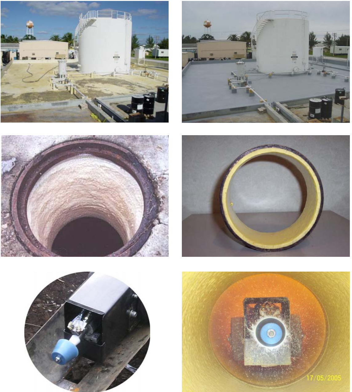
Fig. 1.2. a-f. Polyurea used as concrete coating in a secondary containment: primed (top left) and sprayed the same day (top right). Polyurea used as Manhole rehabilitation: the primed pipe (centre left) and sprayed the same day (centre right). The high pressure spray gun to spray polyurea (bottom). (source: CSI Construction Solution Inc.: Polyurea, 2006)
