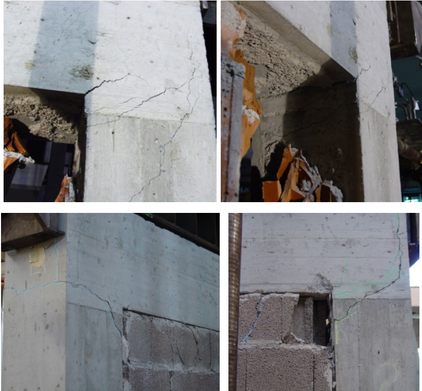
Fig. 2.26. End of column and beam – column joint damaging.
