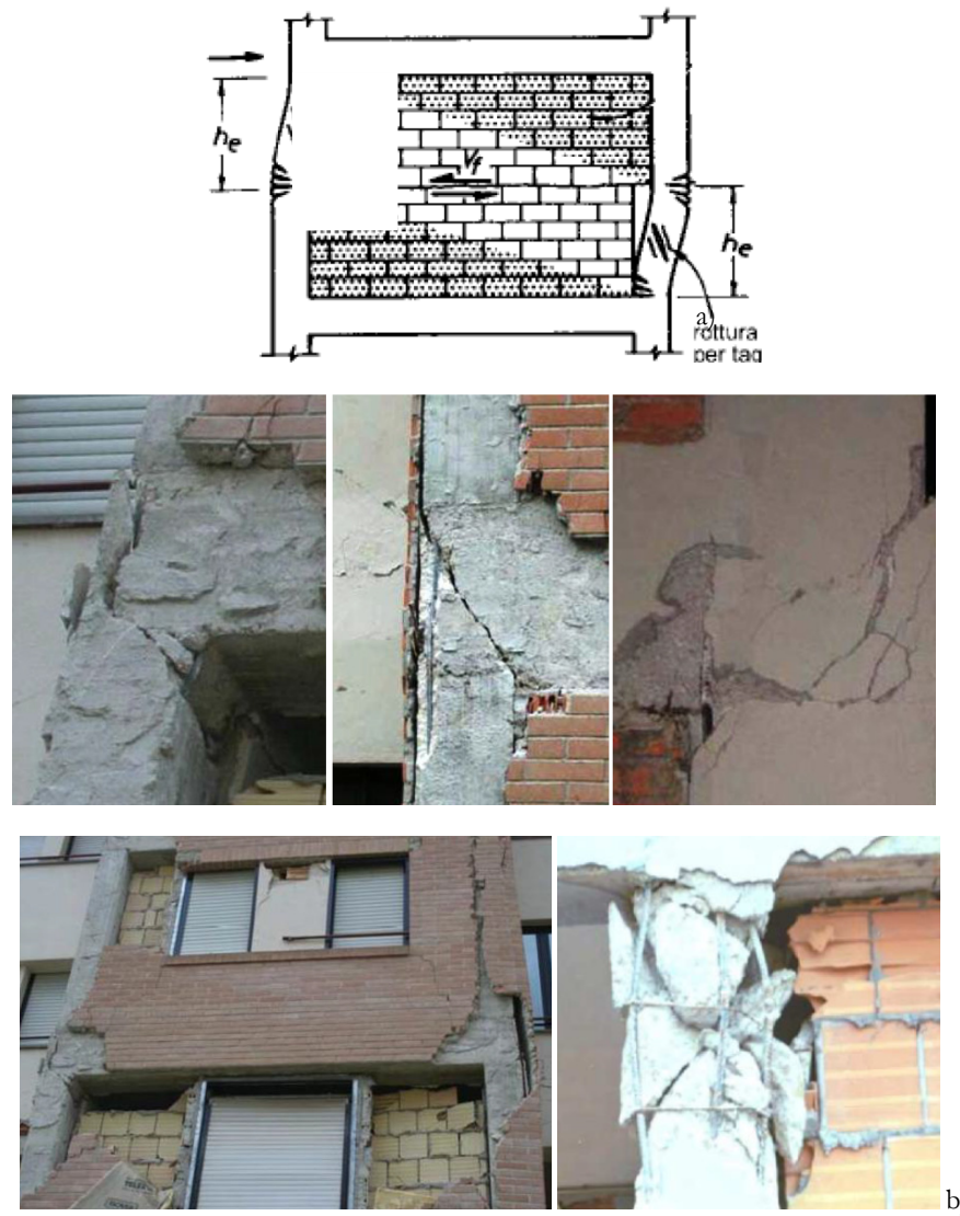
Fig. 1.4. Effects of local infill-frame interaction: a) scheme of collapse mechanism; b) sample of local shear collapse of column ends and joints due to the interaction with the infills.
