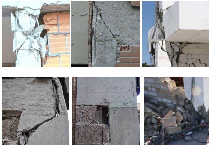
Fig. 4.2. Local shear failure of frames due to interaction with infills under seismic loads.
