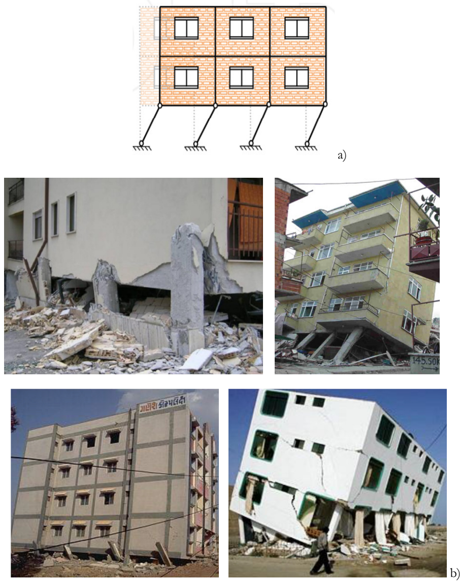
Fig. 1.3. Effects of irregularities in distribution of infills over the height: a) Collapse mechanism; b) Example of collapses occurred for irregular distribution of infills over the height.
