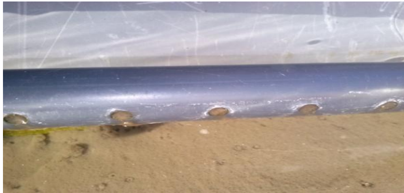
Figure 5.1. Clogging in diffuser
