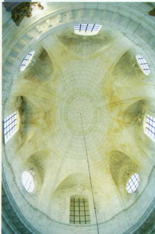
Fig 10: Internal view of the vaults, Chapelle de l'Oratoire, Avignone (Photo by F. Scaduto)
