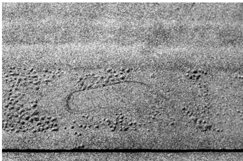
Fig. 2. Low flexibility at low temperatures was not the only problem of asphalts as well as the prefabricated membrane shown in the picture: these first bituminous sheets were made with oxidized natural bitumen or coal tars, stabilized with accurately mixed fillers. Filled oxidized bitumen membranes were much better than natural asphalts and much easier applied than built up roofs, but they still suffered heat: their flexibility were quickly reduced and their melting temperature were still too low. The membrane on the left shows a diffuse blistering and a foot print. Blistering is caused by its water absorbivity, foot-prints by its low melting temperature.
