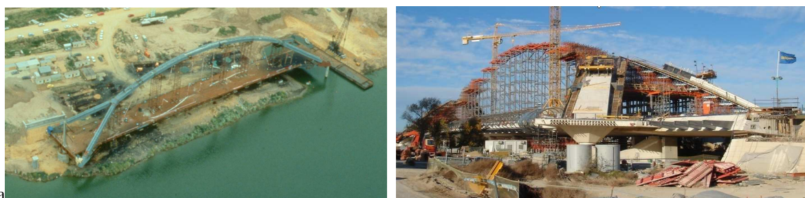
Figure 3. Construction methods. a) Barqueta bridge built on a river side. b) Third Millennium Bridge built on site with the continuous falsework
