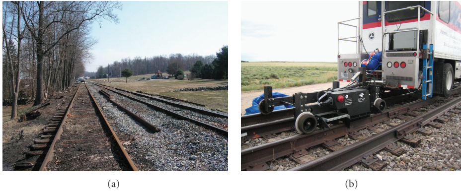
FIGURE 10: (a) Test site near Gettysburg, Pennsylvania. (b) Photo of the latest inspection prototype tested in the field.
