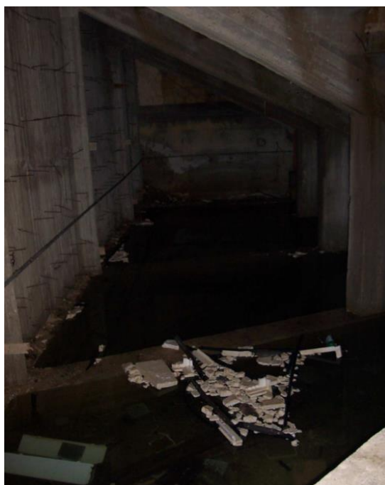
Figure 3. Foundation premises flooded
