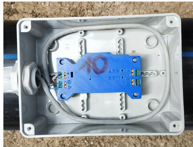
Figure 3 Example of sensor with enclosure glued to the pipe.
