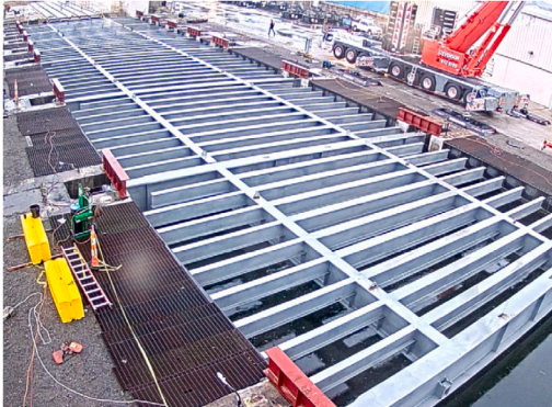
Fig. 1. Structural application of GFRP elements for deck and bridge (photo of the author).
